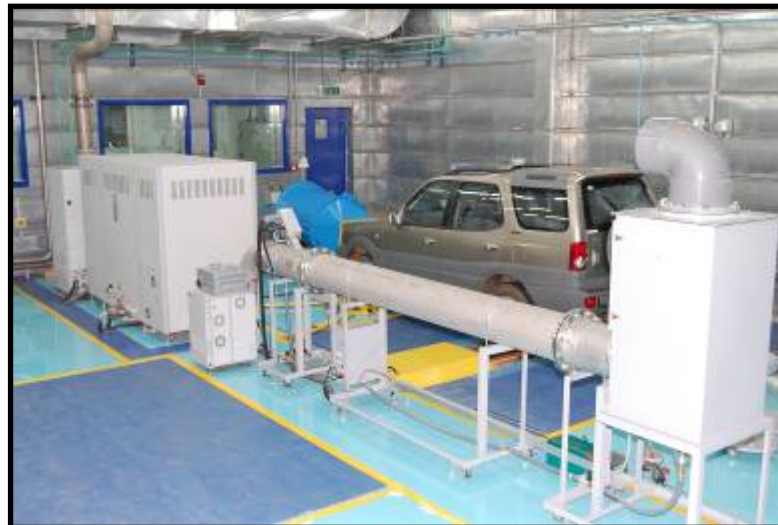
Chassis Dynamometer Test Cell
